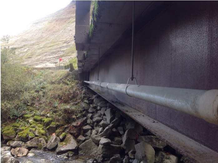
fibre optics line hung from deck panels
