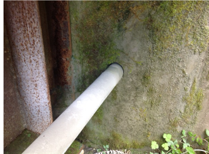
fibre optics line access through ballast wall
