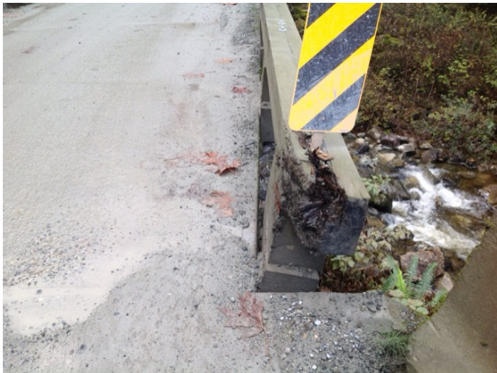
Guard Rail damage
